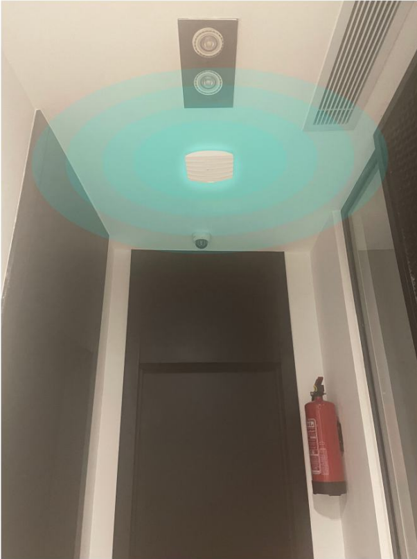
Ceiling-Mounted Access Point (EAP225)
